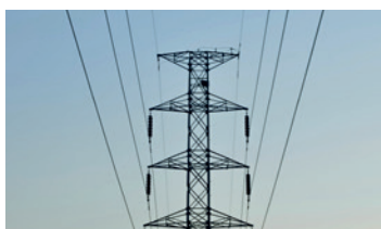
Grid infrastructure (power)
